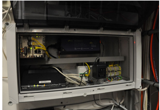
The first unit in the chain of DDW-222's are located in the server room at the east side of the bridge.
